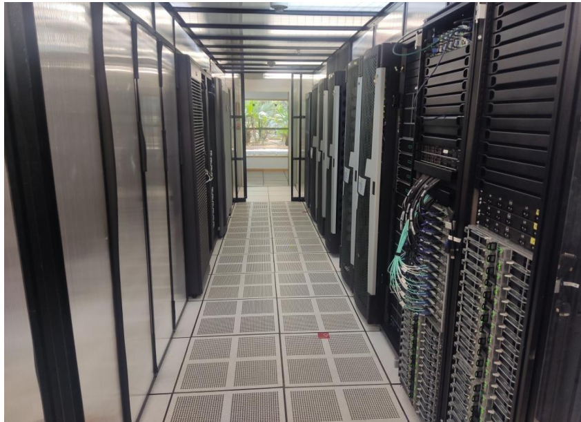
Figura 5.52: Sala cofre II
